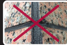
Poor UV resistance - Sealant cracking (PU Sealant)
