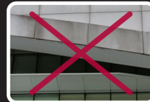
Streaking (Silicone Sealant)
