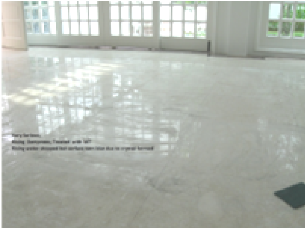
Sealing Rising Dampness
